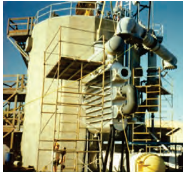
Figure 2. 210 kW Open-Cycle Pilot Plant with Surface Condenser for Water Production. Photo by the author.
